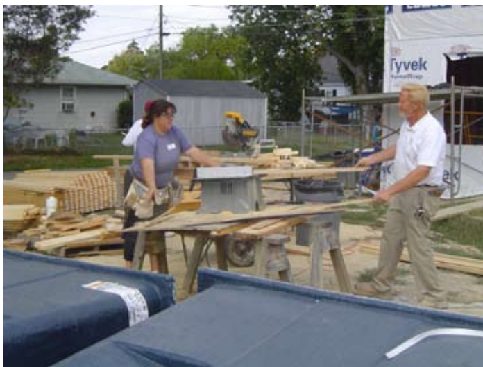
MAERDAF grantee Habitat for Humanity of Talbot and Dorchester Counties was awarded a grant to pay for a full-time construction supervisor, who is credited for helping the organization build five homes that would not otherwise have been built for low income rural families in the area.
